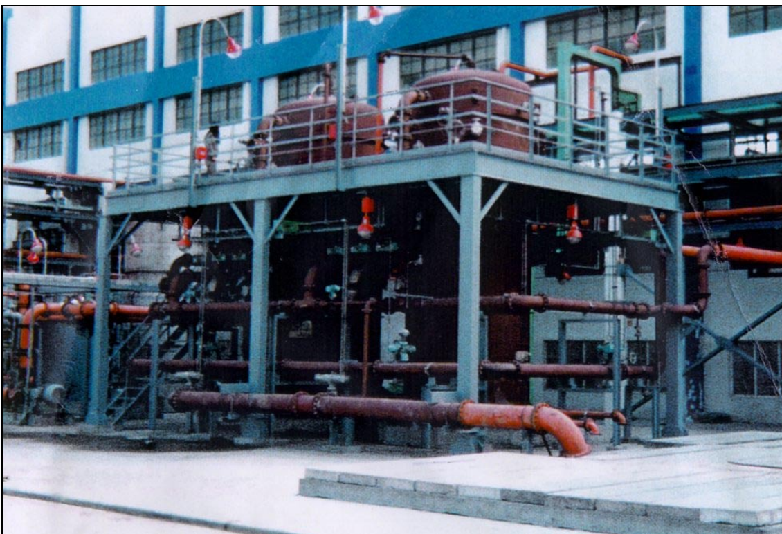
Figure 2.13: View of polishing filters in a secondary brine purification system (photograph supplied by Asahi Glass Co)
