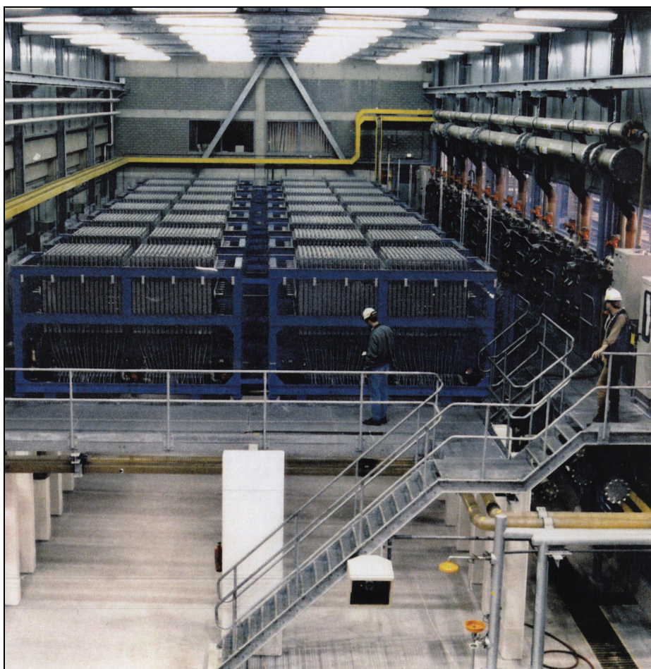
Figure 2.10: View of a membrane cell room equipped with bipolar electrolysers (Source: Hoechst-Uhde)
