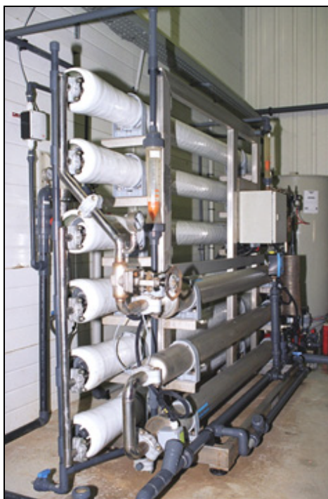
Figure 4.19: Reverse osmosis plant Menoni S.A. and Agence de l'eau Seine-Normandie
