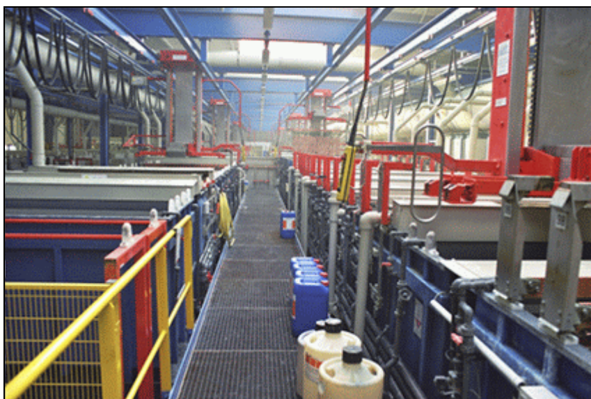
Figure 4.33: Jig line with lids on vats and air extraction Graindorge S.A. and Agence de l'eau Seine-Normandie
