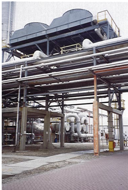
Figure 2.13: Example of a dry air-cooled liquid cooler in a chemical process [Pers. archive]
